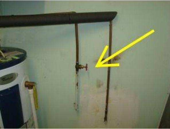
Photo 21-4 Water Heater Shut-Off Valve
