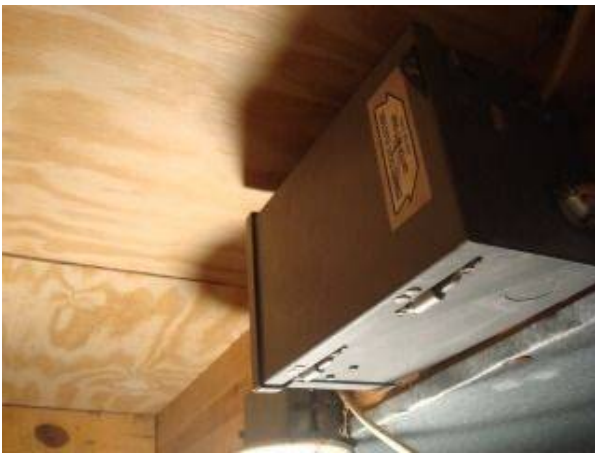
Photo 23-8 Indoor Unit Disconnect
