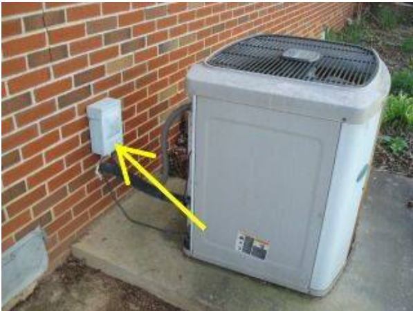
Photo 23-2 Outdoor Unit Disconnect
