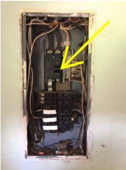
Photo 16-3 Main Breaker Location
